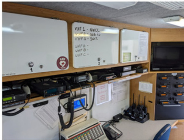
Among the communication gear in the York EMA emergency communications van are banks of VHF, UHF, and HF radios that monitor police, fire, hospital, and school radio systems. All are tied into two redundant consoles allowing up to four dispatchers to work at once if necessary.
